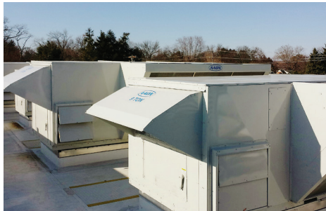
AAON rooftop units
