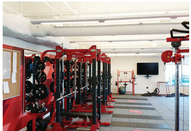
Fitness Center DuctSox
