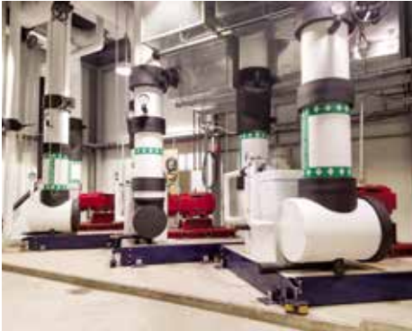
Chilled water pumps.
