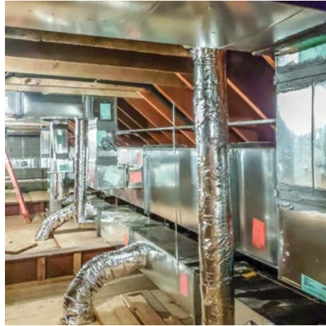
Duct work installed in the church's attic space
