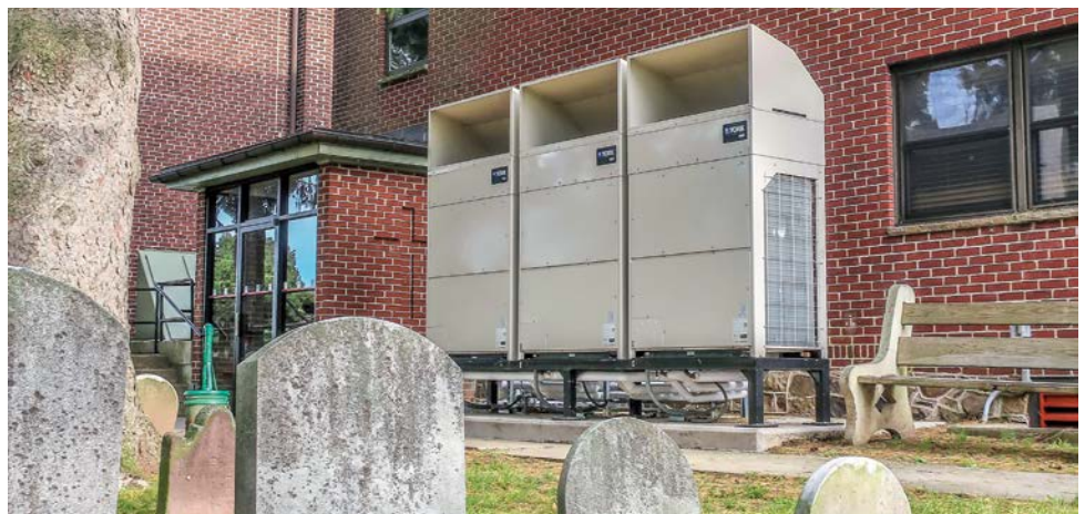
Additional condensing units outside the church
