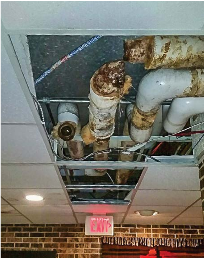
Before: Old piping in the ceiling indicating severe corrosion.
