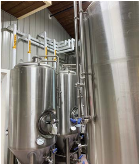
Brew house tanks and piping
