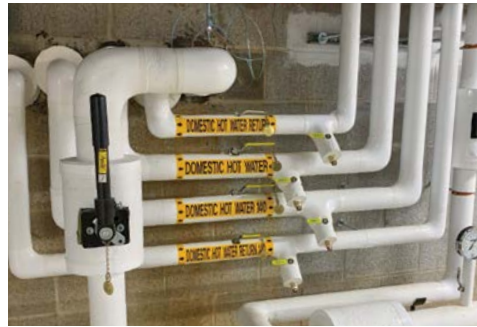
Mechanical room piping
