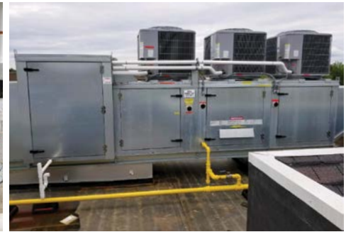
Rooftop mechanical units
