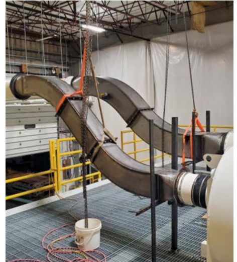
Scrap system intake duct
