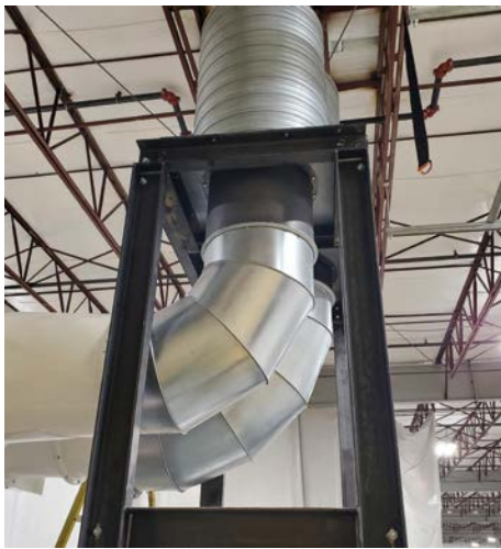
Scrap system exhaust duct
