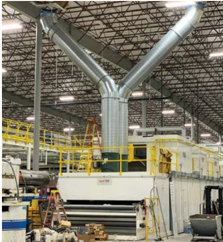
Intake and exhaust duct
