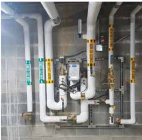
Mixing valve station
