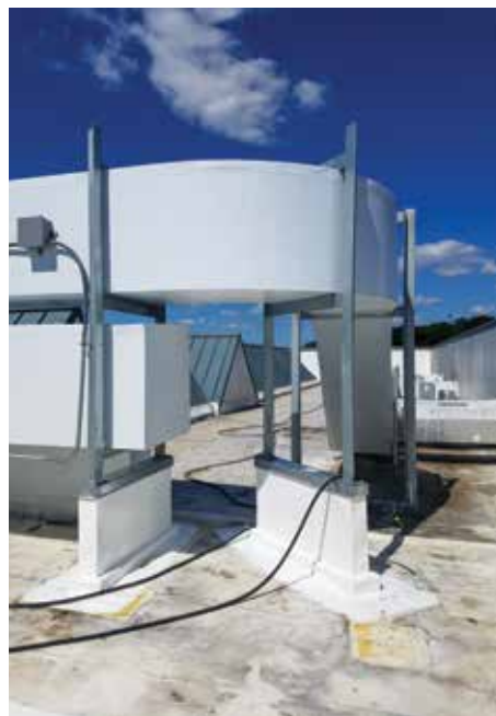
Rooftop ductwork supports
