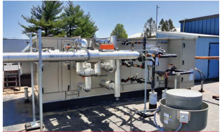
Rooftop Air Handler
