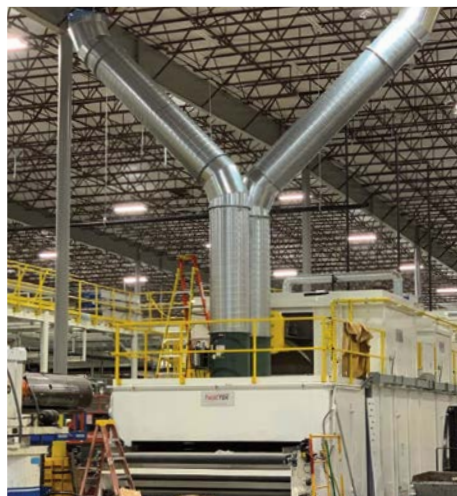
Intake and exhaust duct
