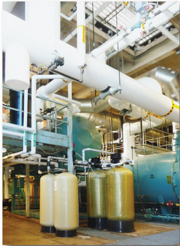
Water softener and deaerator.
