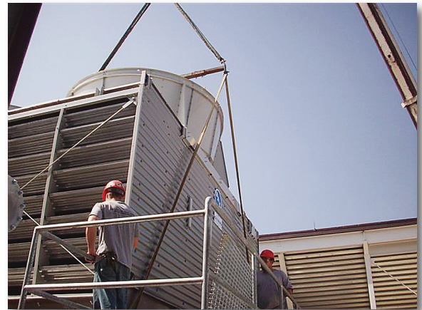
Cooling tower set in place.
