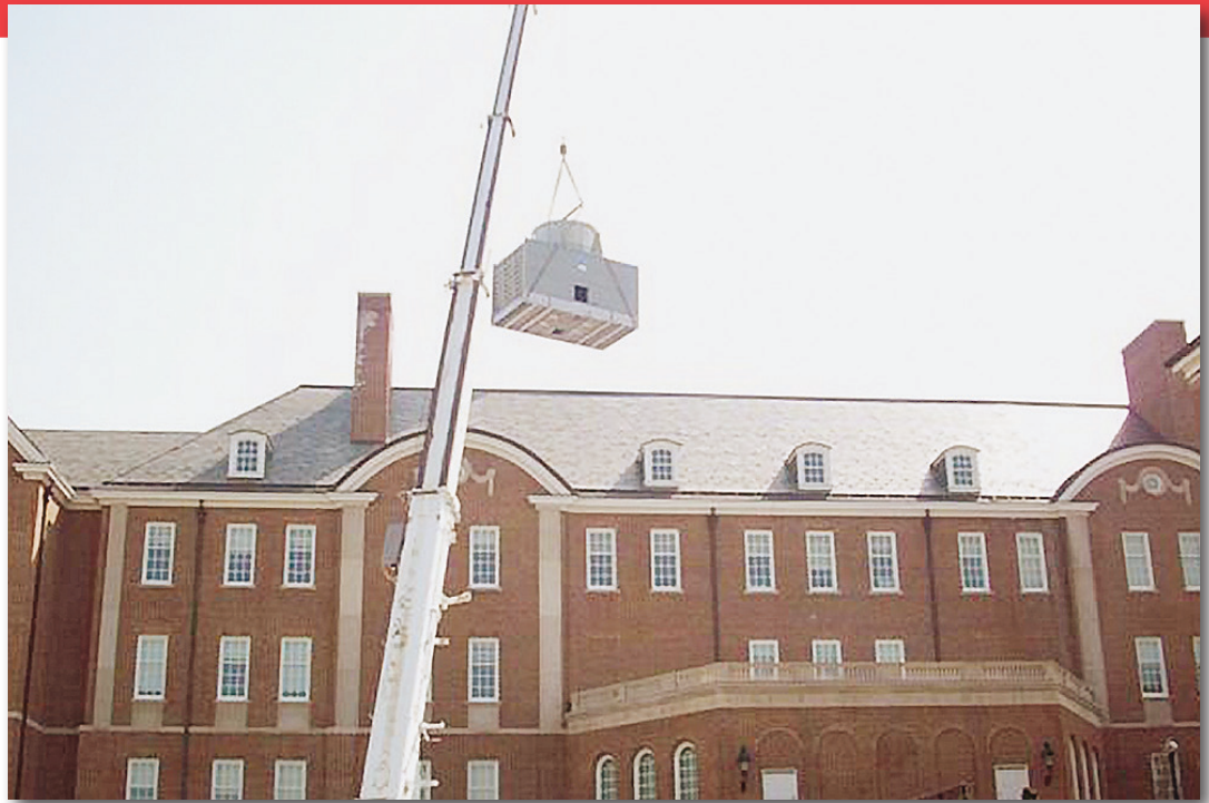
Setting the new chiller in place presented a significant challenge. Pictured above, the cooling tower gets lifted into place.
