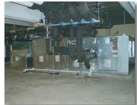
The basement air handler.
