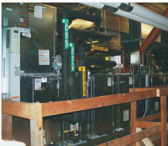
The attic air handler.
