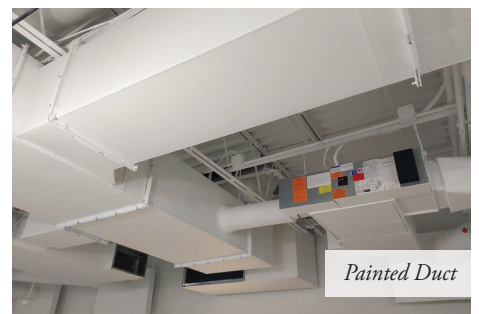
Rectangular & Spiral Duct
